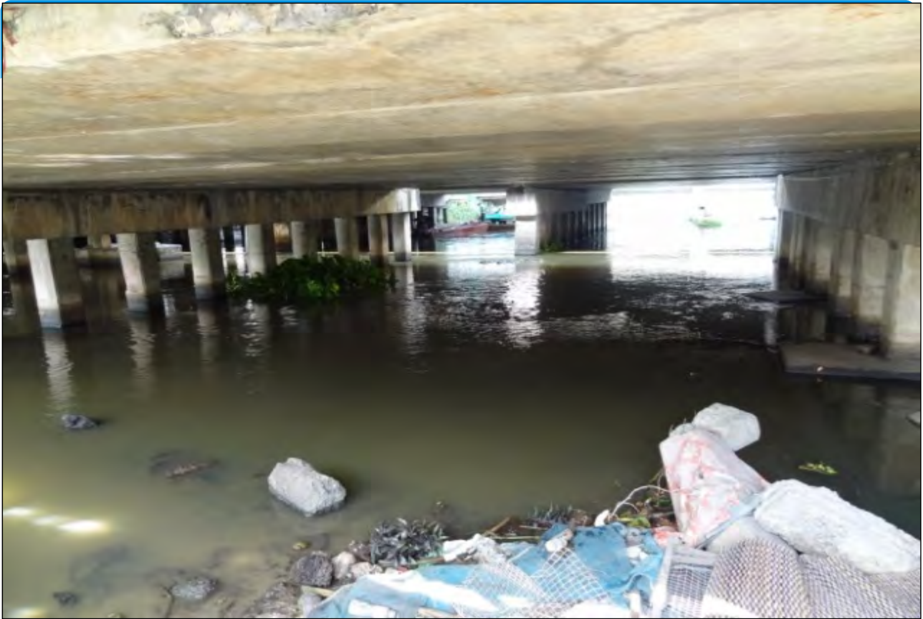
Uncleared and wrong alignment of Bridge support
