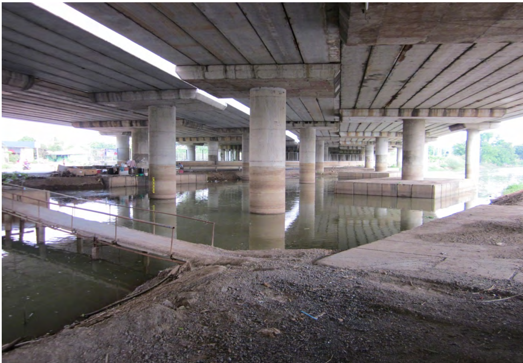
Bridge footing obstruct channel flow
