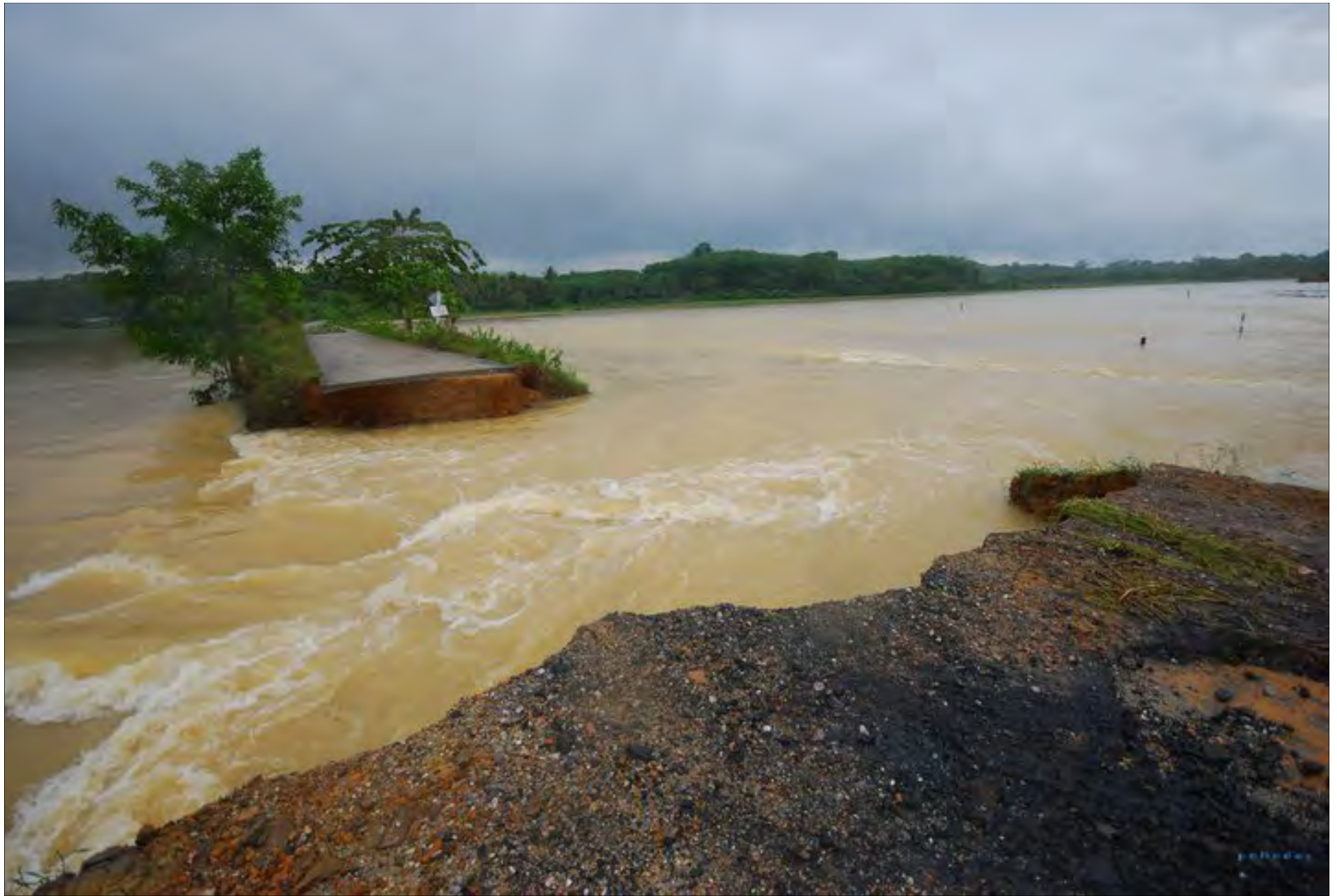
Road obstructing surface run-off
