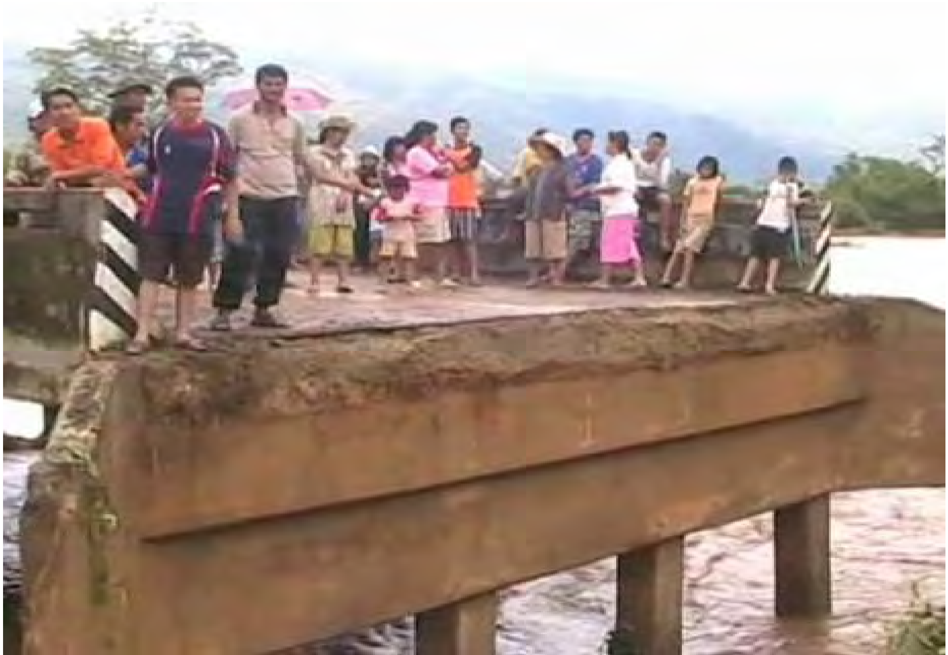
Inappropriate design of Bridge Abutment
