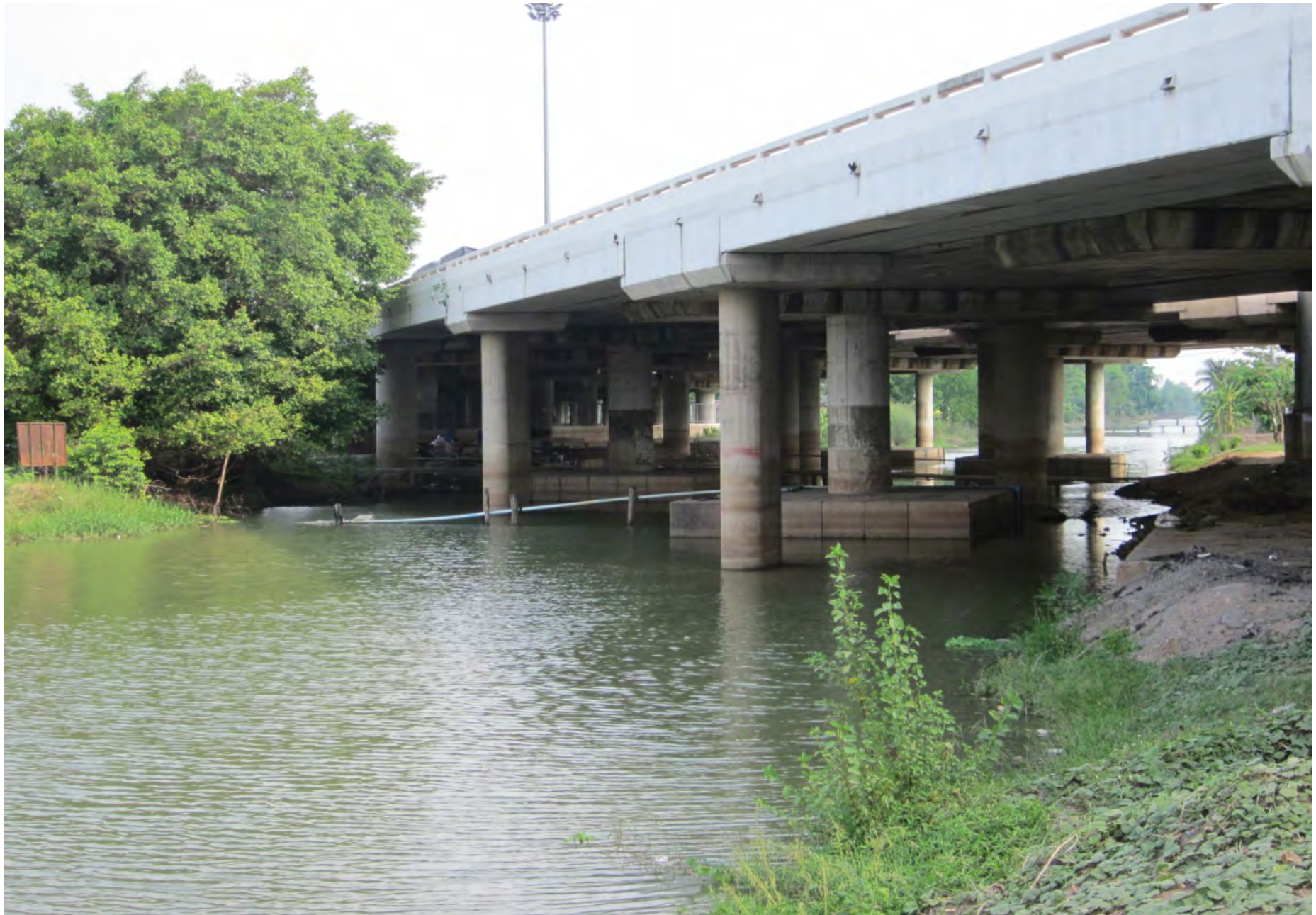
Bridge footing obstruct channel flow
