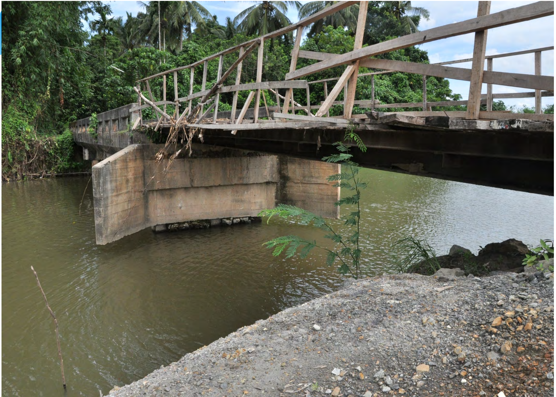
Inappropriate design of Bridge Abutment
