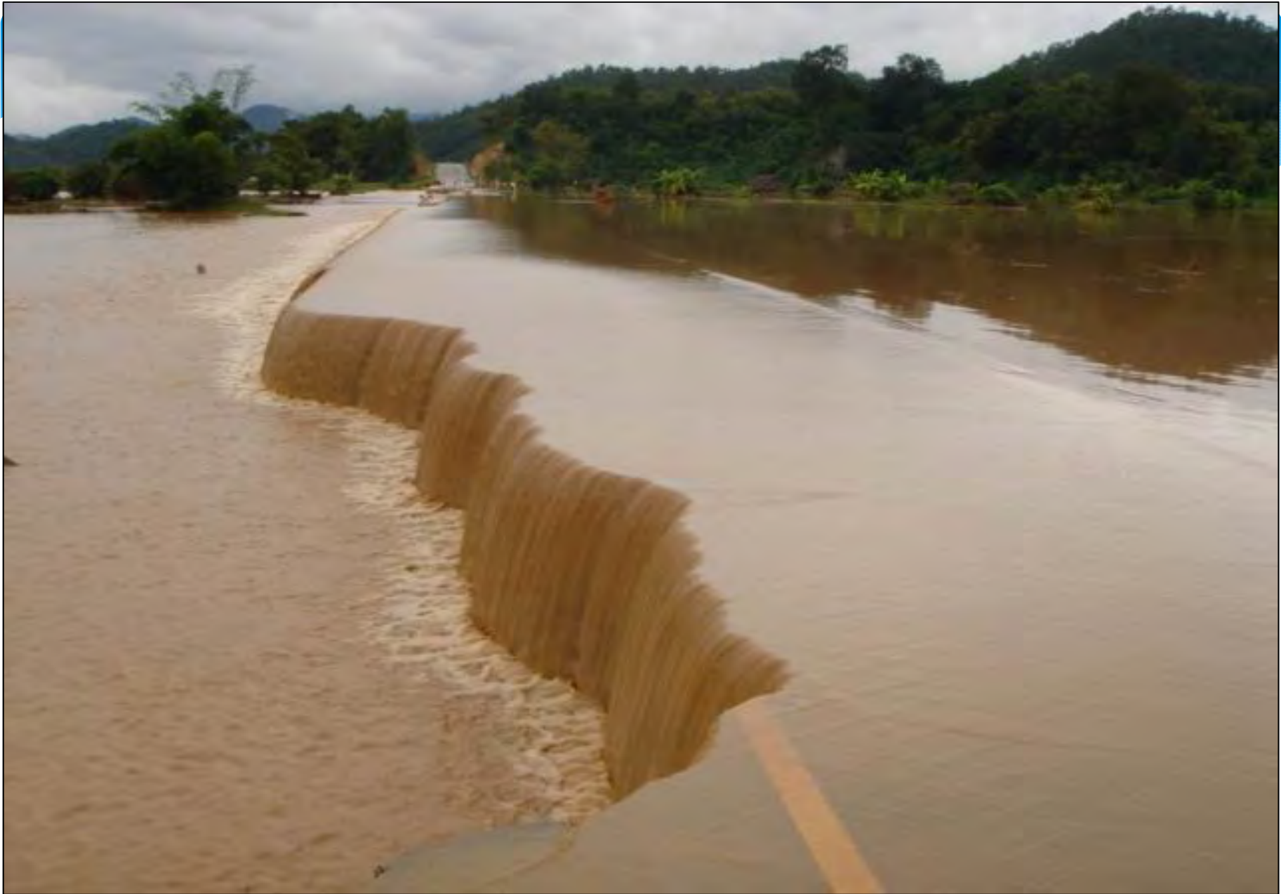
Road obstructing surface run-off
